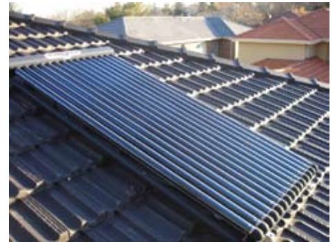
Solar evacuated tube hot water system.
